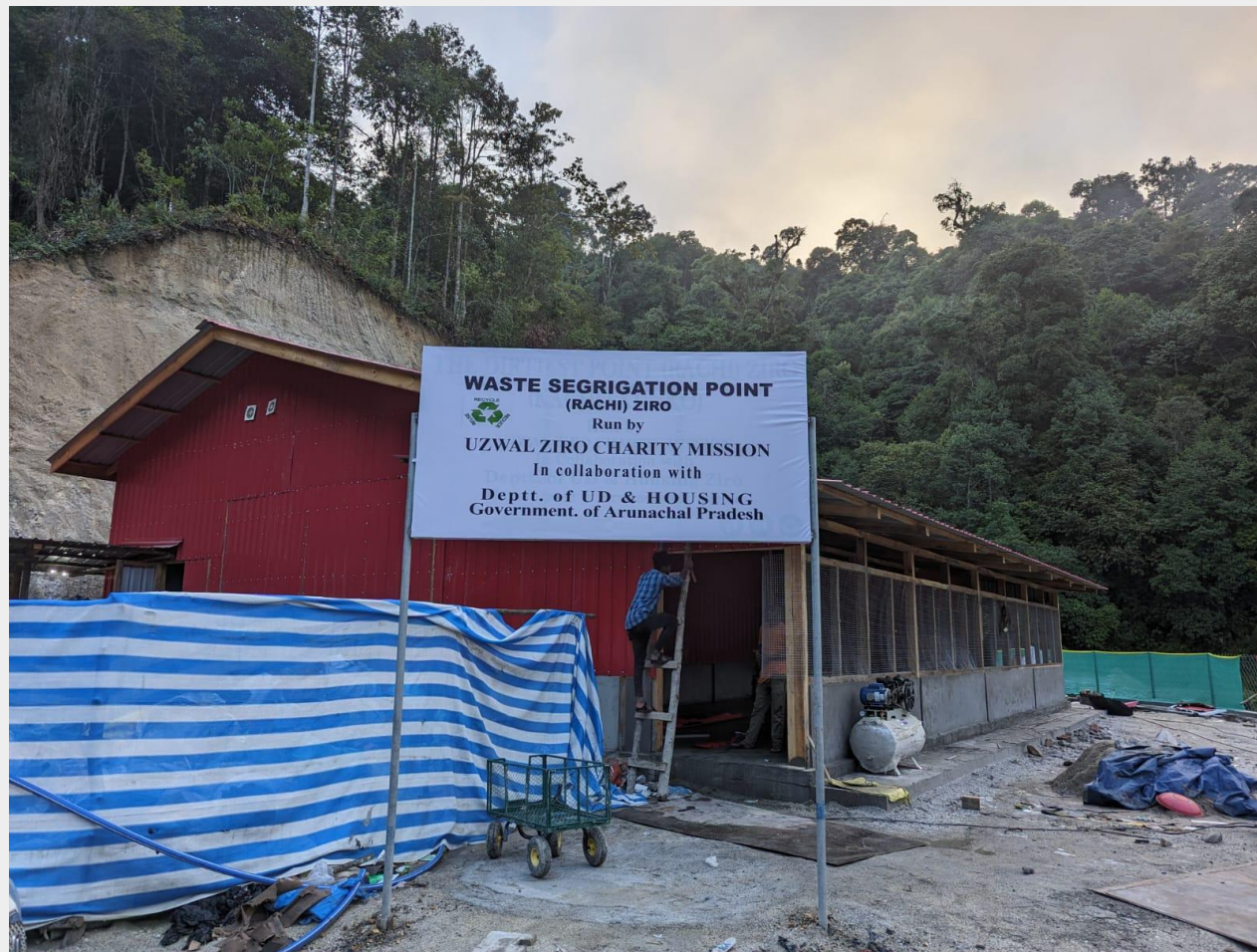
Uzwal Ziro Charity Mission's waste segregation facility located on the outskirts of Ziro
