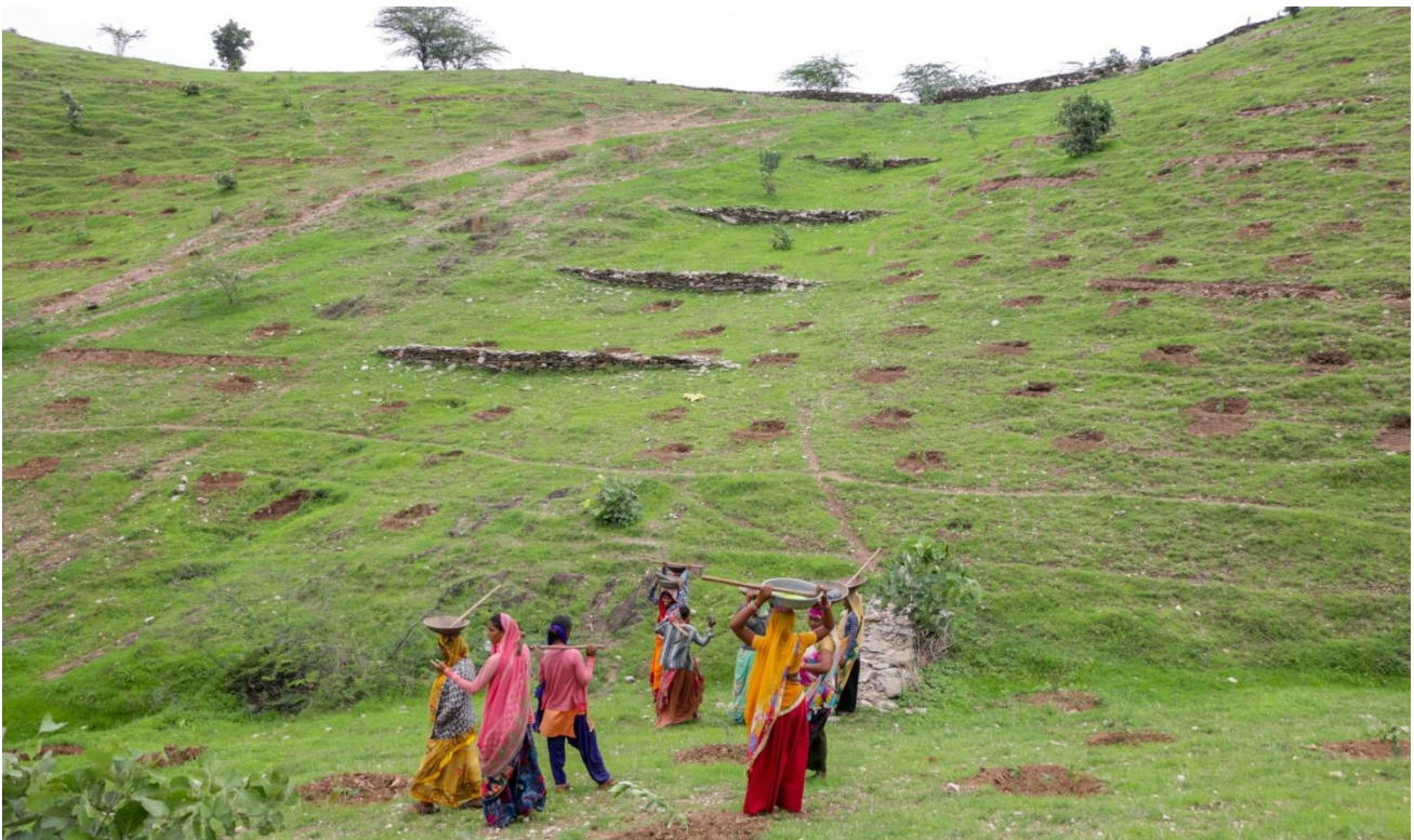
Newly constructed gully plugs on a pasture land in Kherwara to restrict rain water run-off
