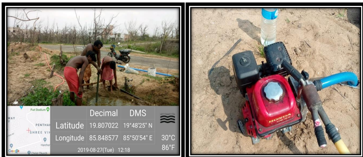
8 PUMP-BASED BORING SYSTEM FOR SUFFICIENT WATER SUPPLY FOR THE PLANTS
