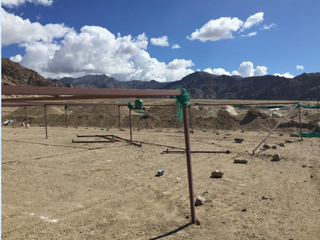
Figure 10. Nursery frame damaged by wind after shade net was blown off. Photo from August 29 th .
