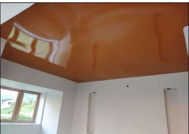
Work of false ceilings and interiors completed in the six homestays of Makkumath
