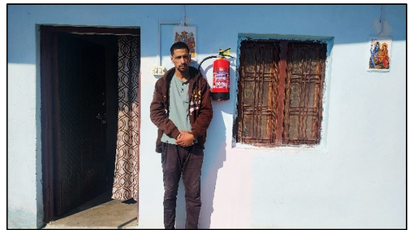
Fire Extinguishers installed in Jadipani HSs
